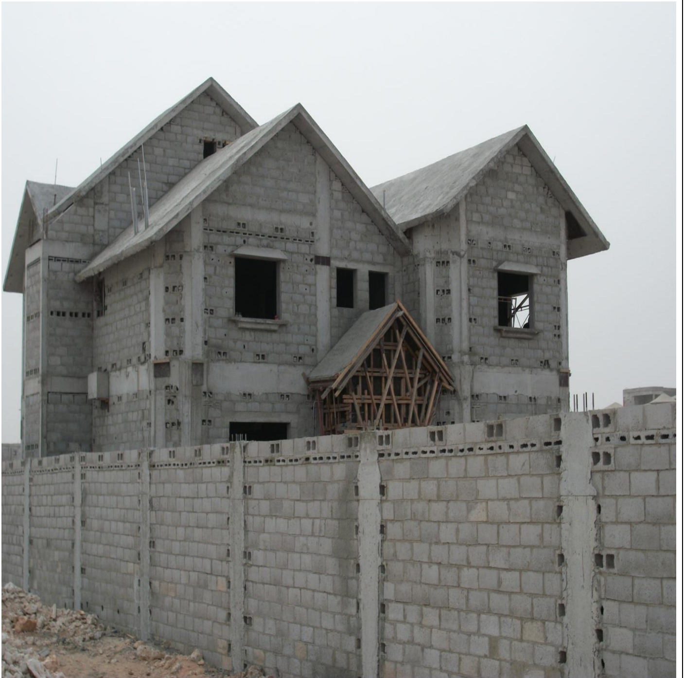
Construction of G+1+1 Villa for Mr. Rashid Ramadan F. AL. Ali at Ain Khalid
