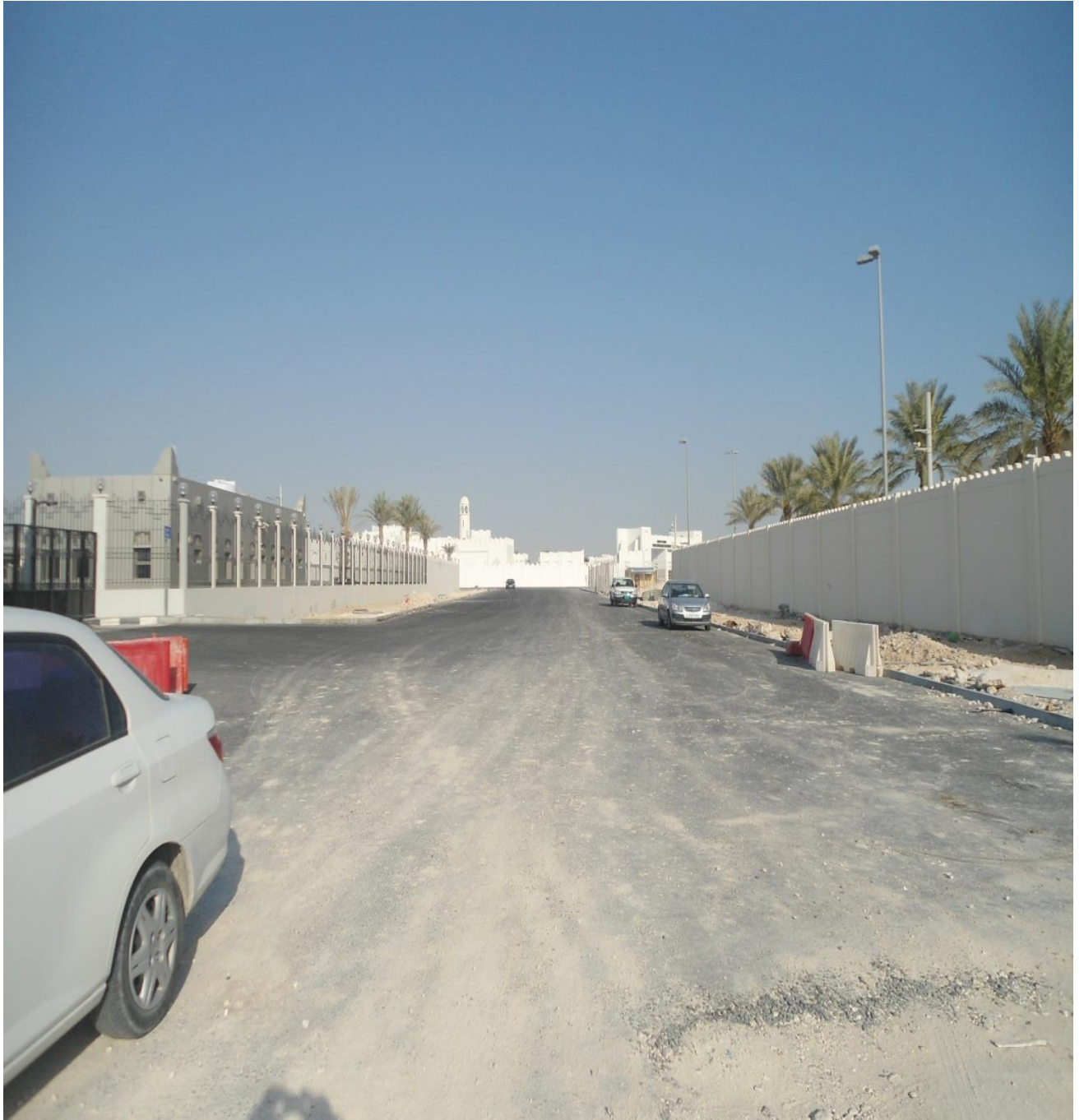
CONSTRUCTION OF INTERNAL LINK OF INFRASTRUCTURE AND LANDSCAPING FOR MOI PROJECT AT DUHAIL ROAD D2 AND D4
