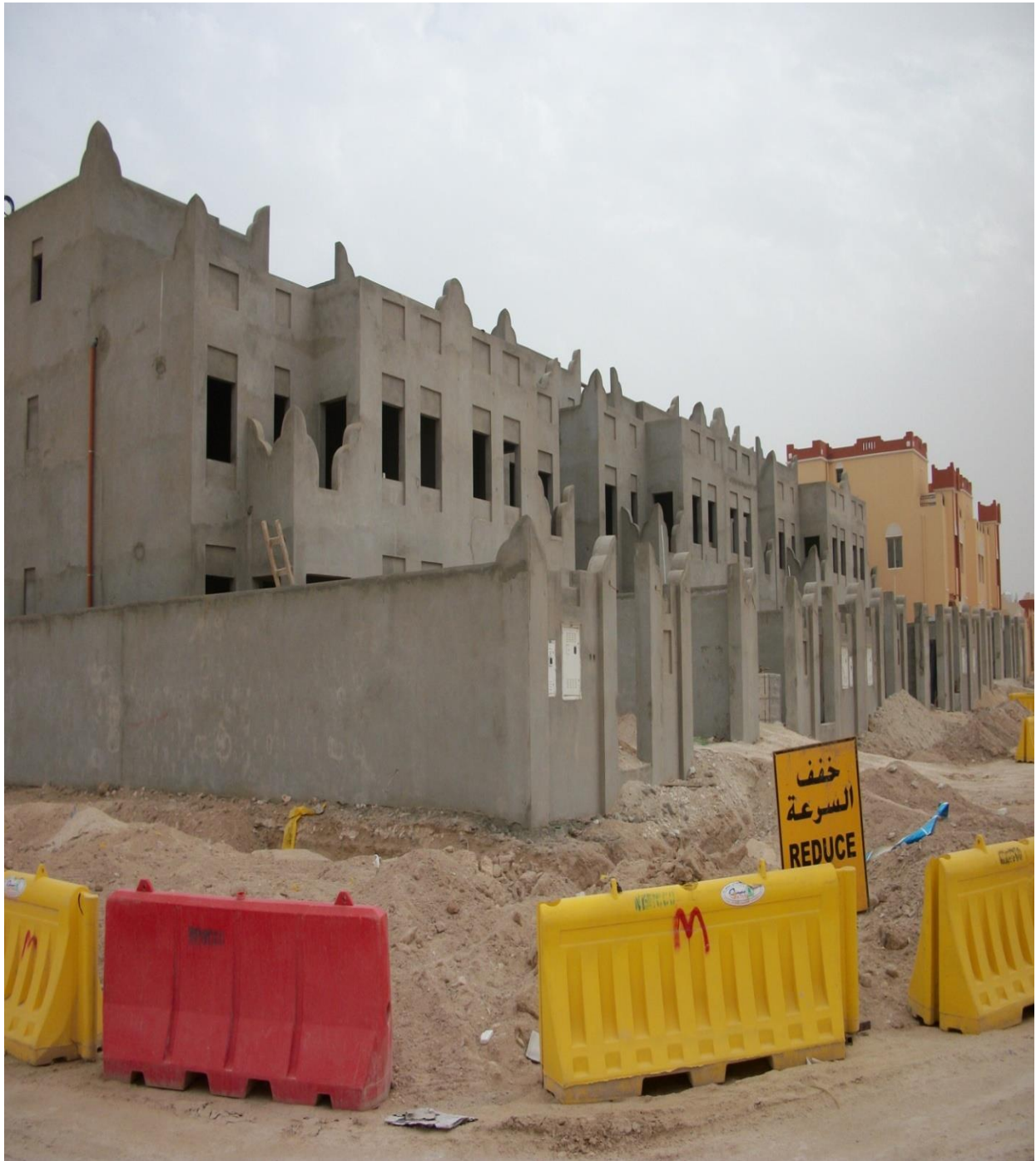
Construction of 12 Nos G+1+P villa at Gharaffa for Sheikh Fahad Bin Thani Al Thani
